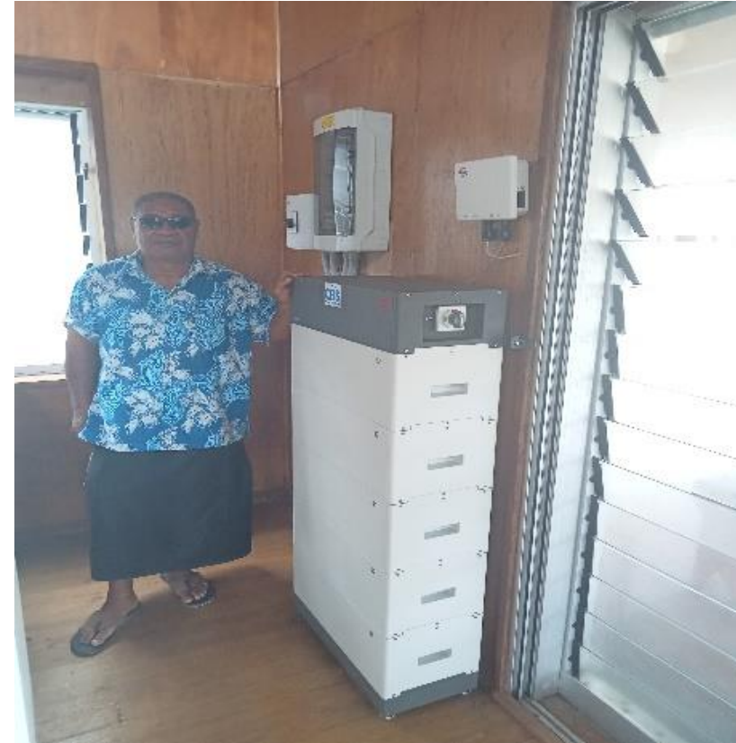
20kWh lithium-ion battery
