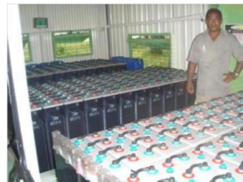
Battery Bank in Vaitupu
