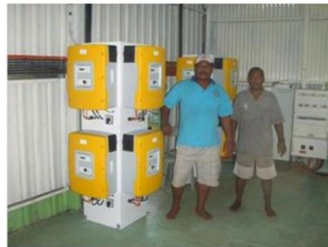
Battery Controls in Vaitupu (SMA)
