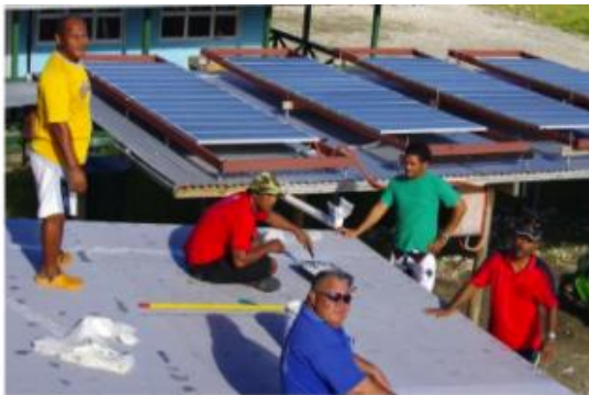
TEC staff installing a non-metallic, low maintenance and cyclone proof demonstration solar roof
