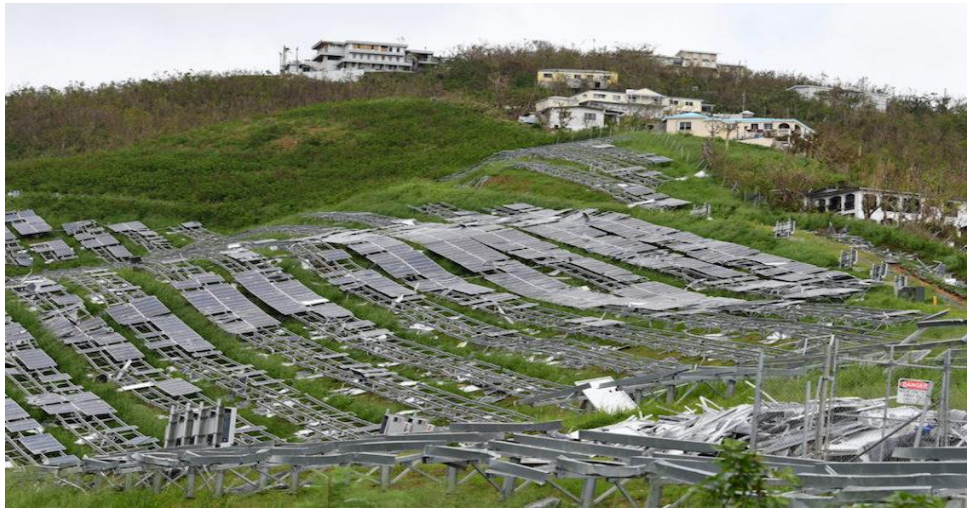
Damage to St Thomas PV plant after Hurricane IRMA (VIRGIN ISLANDS - Caribbean Sea - US – SEPT 2017) (Source: “Solar under storm” – Rocky Mountain Institute)
