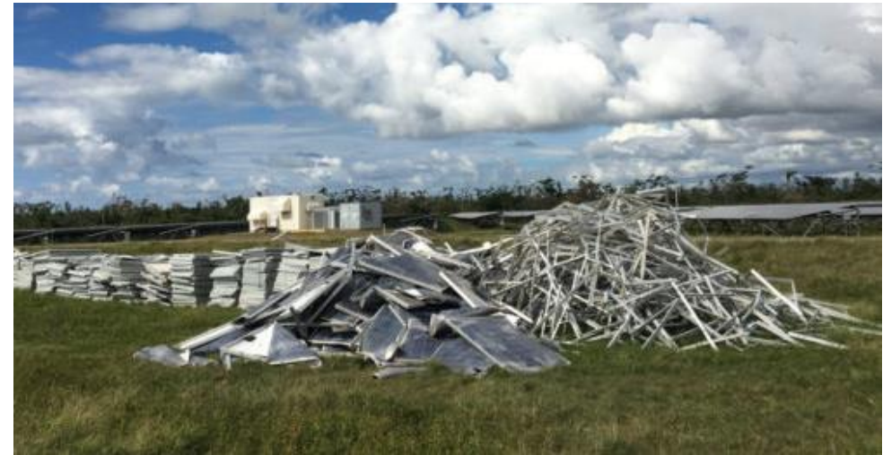
Damage to Illumina PV plant (24MWp) after Hurricane MARIA (PUERTO RICO in 2018) (Source: Maria Gallucci/IEEE Spectrum)
